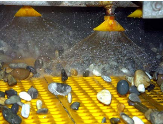
Water washing process for aggregates – UNICEM
