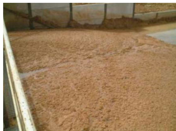
Sludge concrete forced with flocculants decantation cells – Sand and gravel pit – FdA – Spain
