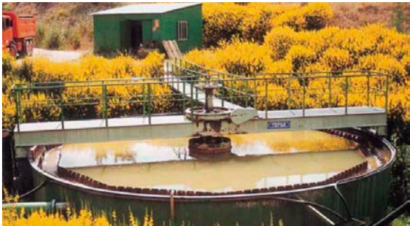
Thickening tank – Sand and gravel pit – Valdocarros site – Tramsa – Spain
