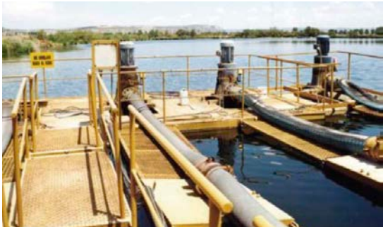
Pumping system for cleaned water – El Porcal site – Aripresa – Spain
